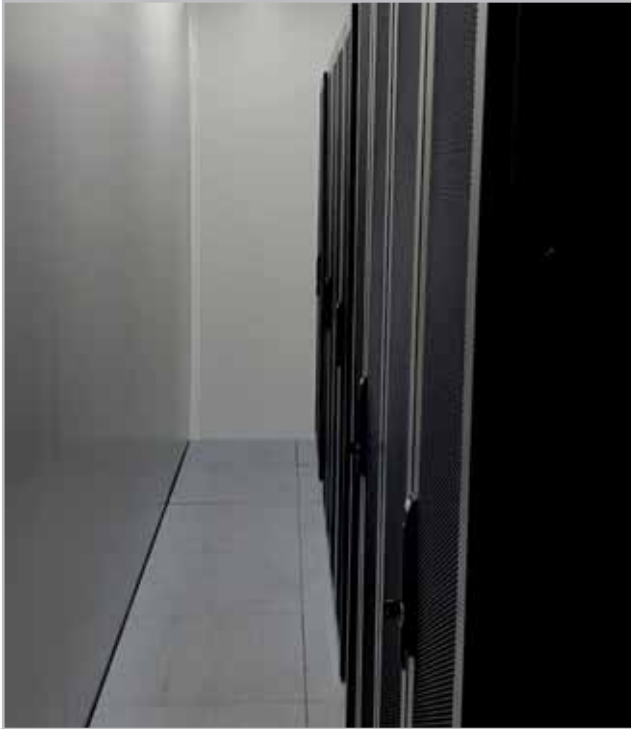
Corridor behind BKT4DC RACKS
