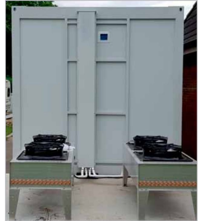
Condensers of BKTinROW cooling ready to work
