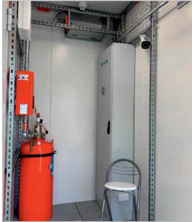
Technical room space: Fire&Exting.sys., container main switchboard
