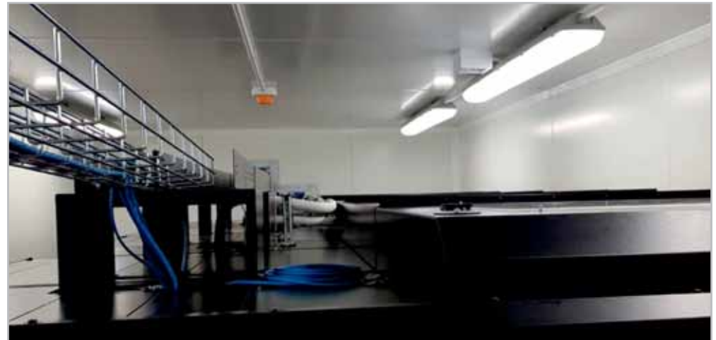
Installation of cable trays, BKT4DC ducts, installation of a cold aisle system and laying LAN cables
